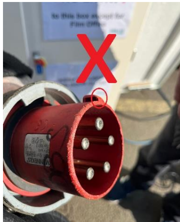
Plug is worn/ damaged.
