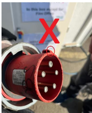
Plug is warn/ damaged.
